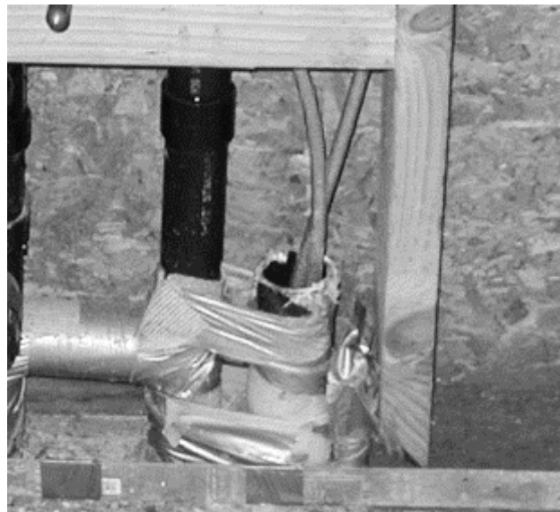
Figure 11-72: Noncompliant Below-Grade Piping and Hot and Cold Water Lines Separation
