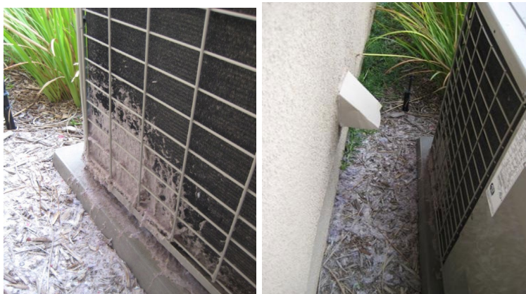
Figure 11-35: Noncompliant Condensing Unit Clearance from Dryer Vents
