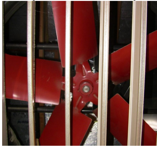
Figure 4-39: Open Barometric Damper With Fan Above
