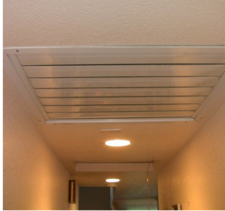
Figure 4-38: Whole-House Fan With Barometric Damper
