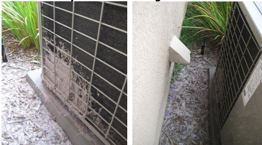
Figure 4-2: Noncompliant Condensing Unit Clearance from Dryer Vents
