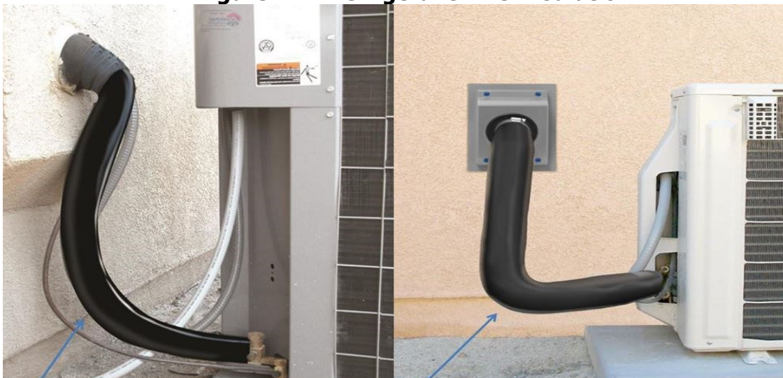
Figure 4-1: Refrigerant Line Insulation
