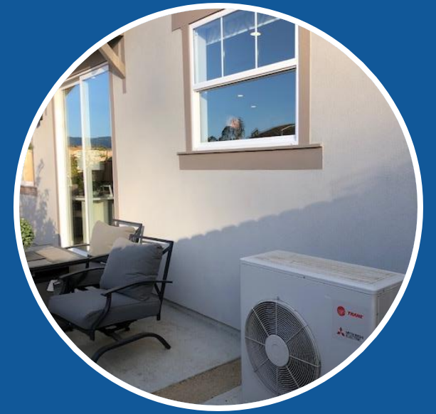
Heat Pump Condenser
