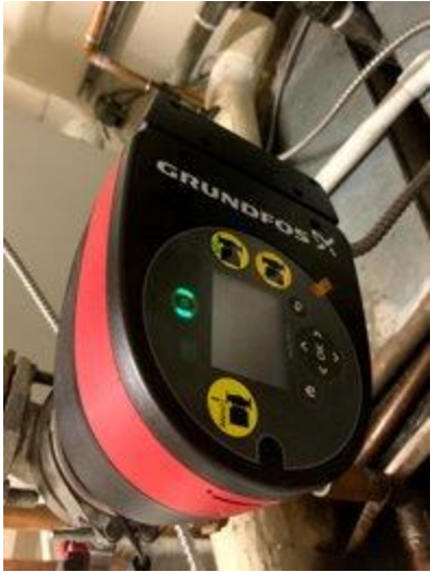
Variable speed recirculation pump with temperature-based controls
