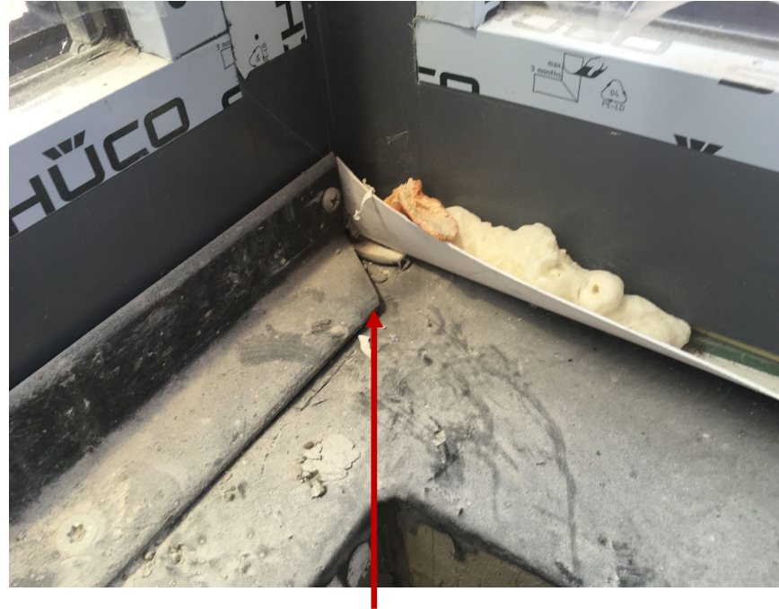
Unacceptable install conditions. No way to guarantee an airtight seal.
