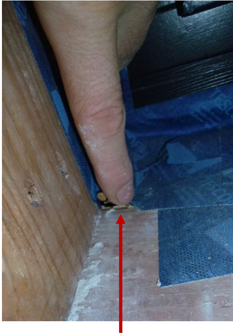
Tape is delaminating because it was applied to a dirty surface!
