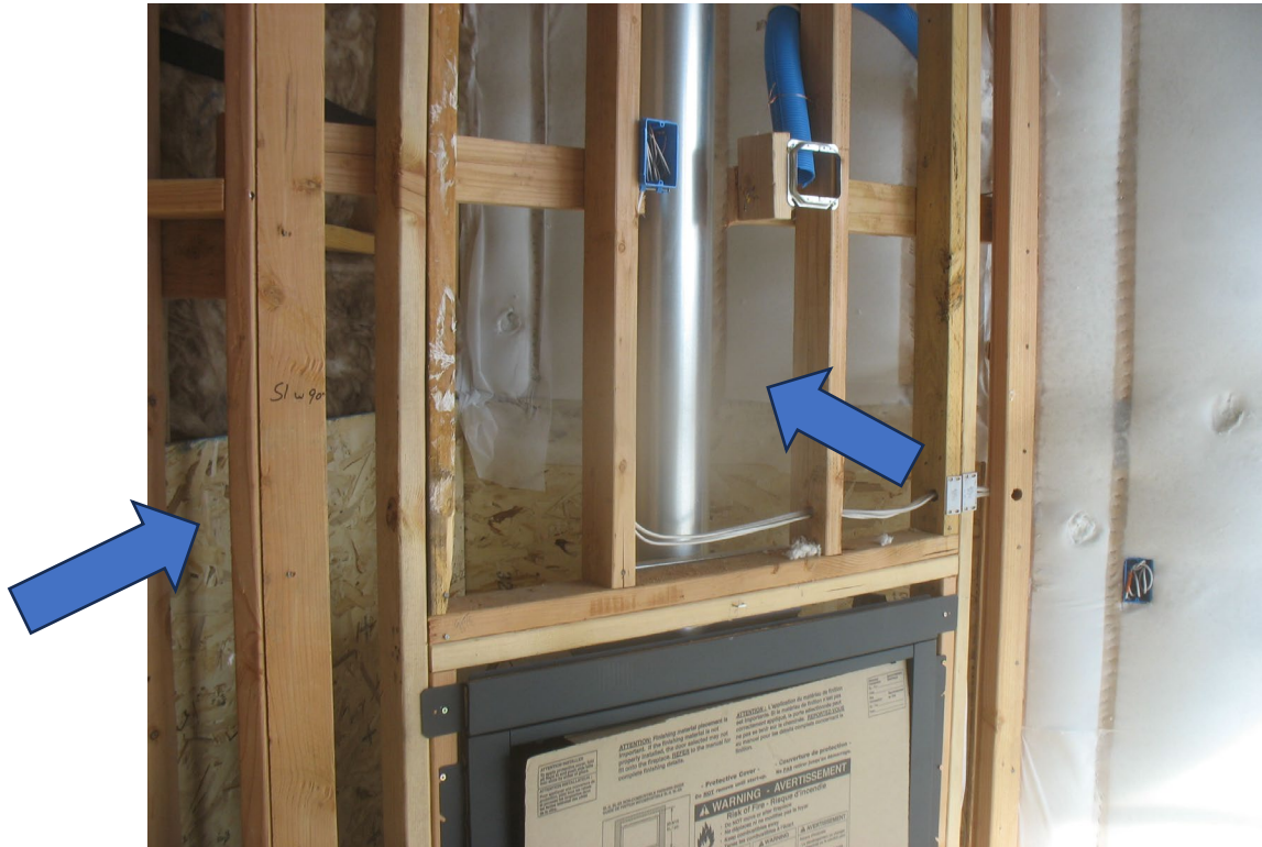
Insulation was blow-in behind the OSB panels. Note: The proper air-barrier is at the exterior walls, not the fireplace surface.
