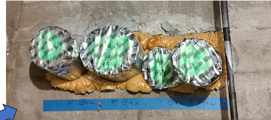
Conditioned 'Daylit' Basement to Crawl Space – Penetrations are air sealed and walls will be insulated.
