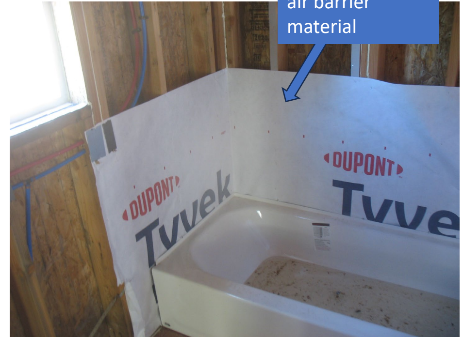
Proper insulation and air-barrier missing behind tub at the exterior walls.
