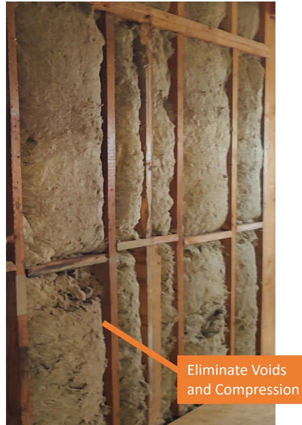
Insulation was compressed at the framing members.
