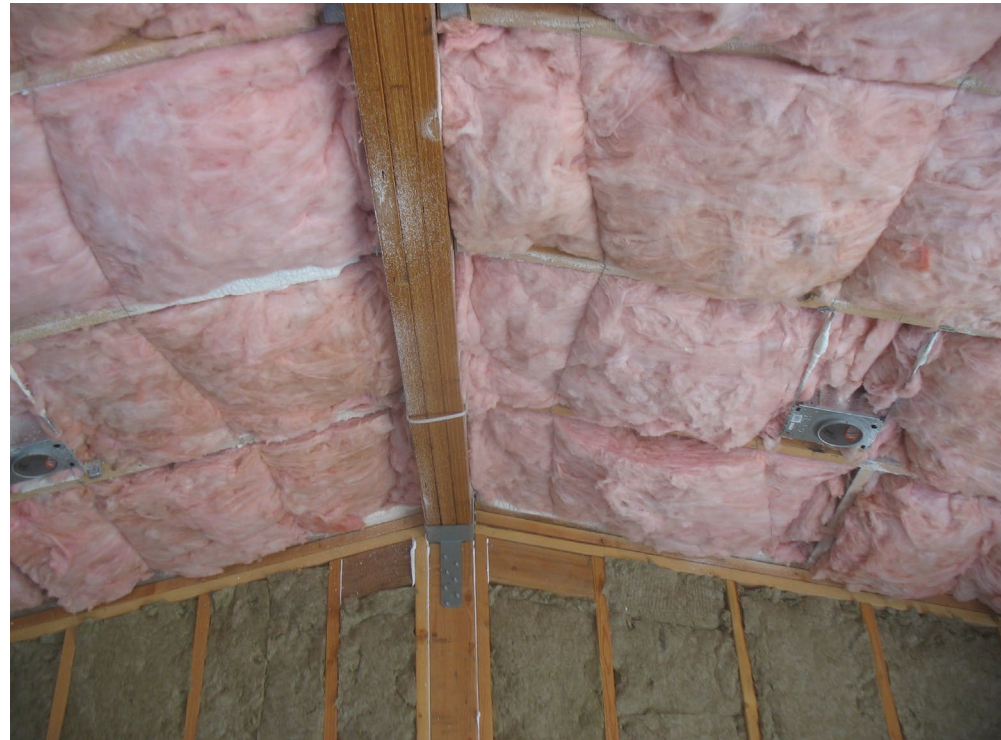
Remaining cavity is filled with Batt Insulation. (Blown-in insulation would also be acceptable.)
