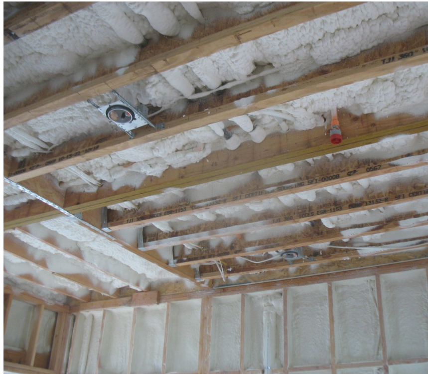
2" Closed Cell Spray Foam is adhered to underside of roof deck and walls.
