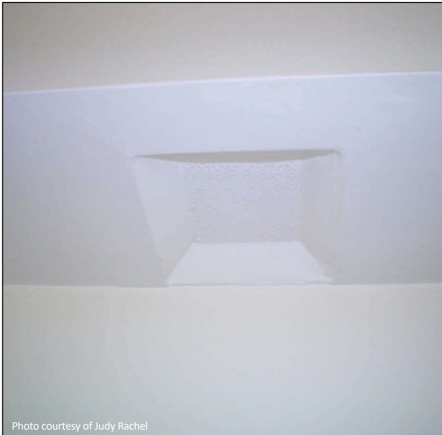
Passive Kitchen Ventilation blocked off but replaced with nothing
