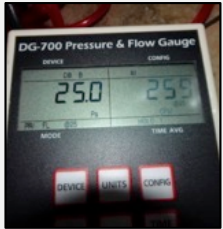
Total Duct Leakage
