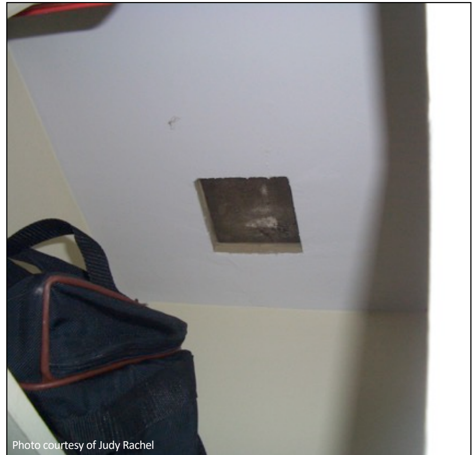
Passive closet ventilation into attic
