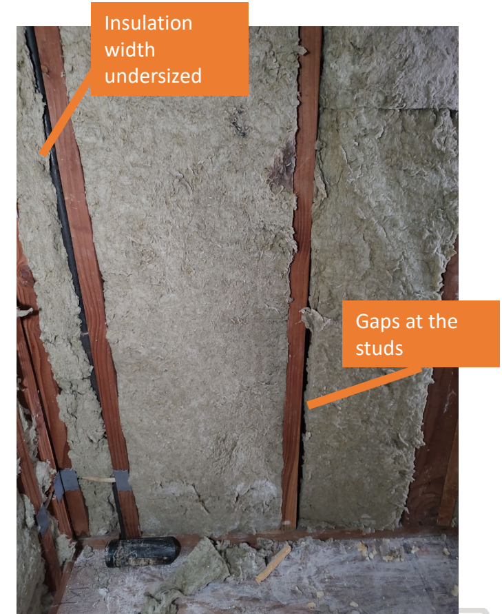
Insulation needs to be in tight contact with the studs.
