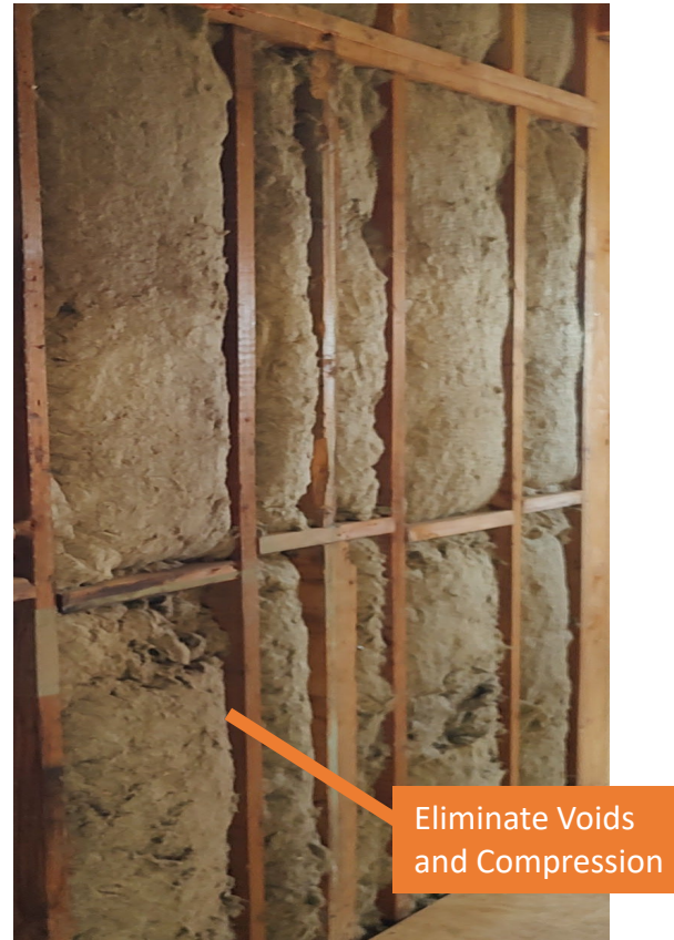
Insulation was compressed at the framing members.
