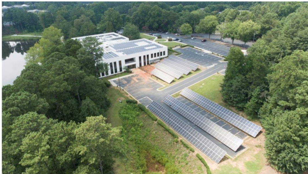
ASHRAE's recently installed photovoltaic (PV) system.
