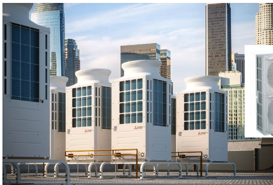
Centralized Air -Source Heat Pumps With Distribution Zones
