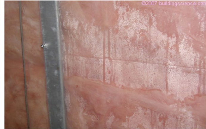
Interior Polyethylene Vapor Barrier – Condensation from inwardly driven moisture
