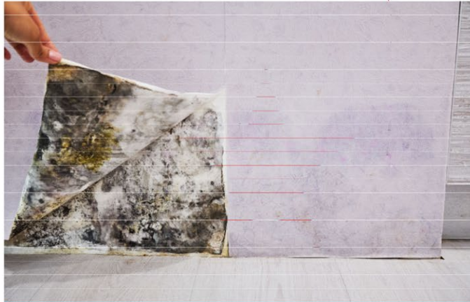
Vinyl Wallcovering – Mold due to inwardly driven moisture trapped by the vapor impermeability of the vinyl wallcovering
