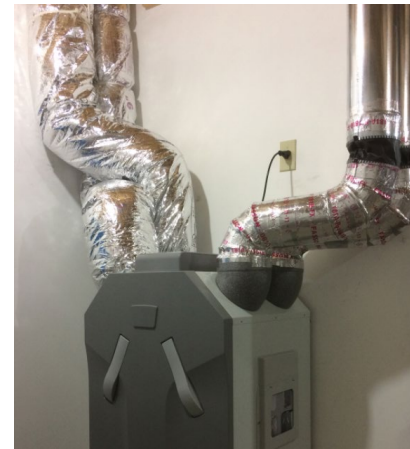
Intake and exhaust duct insulation
