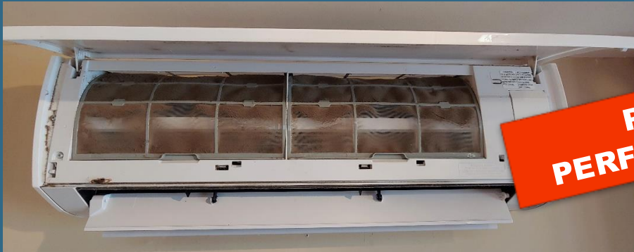
Under the Hood –with dirty Filters
