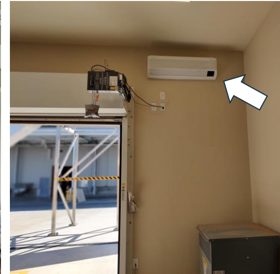
Work Room – ductless wall mount unit
