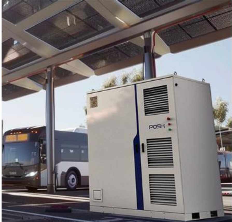
Stanford University EV Bus Fleet Solar with Battery Storage
