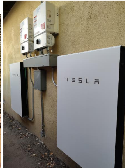
Battery Storage: Two batteries are providing whole home back-up – for the most part...
